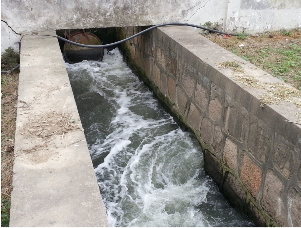
Figure 14. Tongxin North pumping station discharge channel. Dark colored water is pumped from the Louxia River into the Hanpu River
