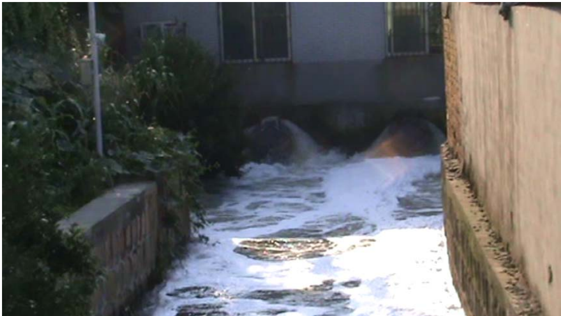
Figure 8. Water being discharged from the Foxconn pumping station
